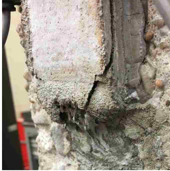
Figure 4.10. Longitudinal crack propagation into end anchorage at failure (specimen DS_330_50_E_4)
